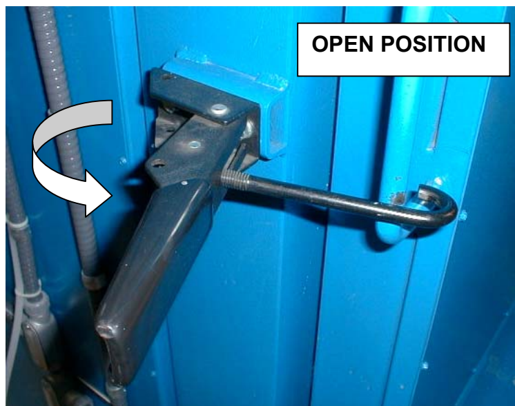
Fig. 3 - 3: Cabinet Door Latch
