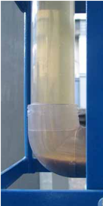
Settled floc in the Site Glass
